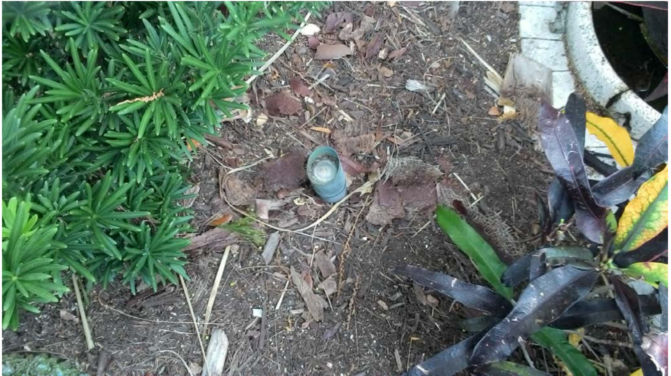
Lighting - Pool Deck
