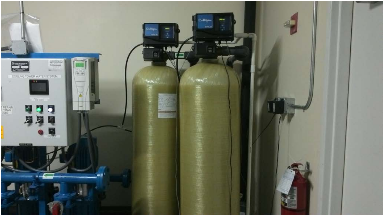
Water Softener - Cooling Tower
