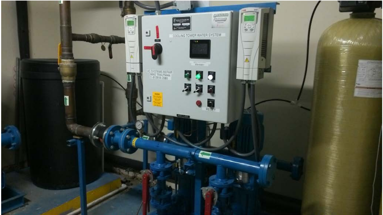
Cooling Tower Drain Pumps
