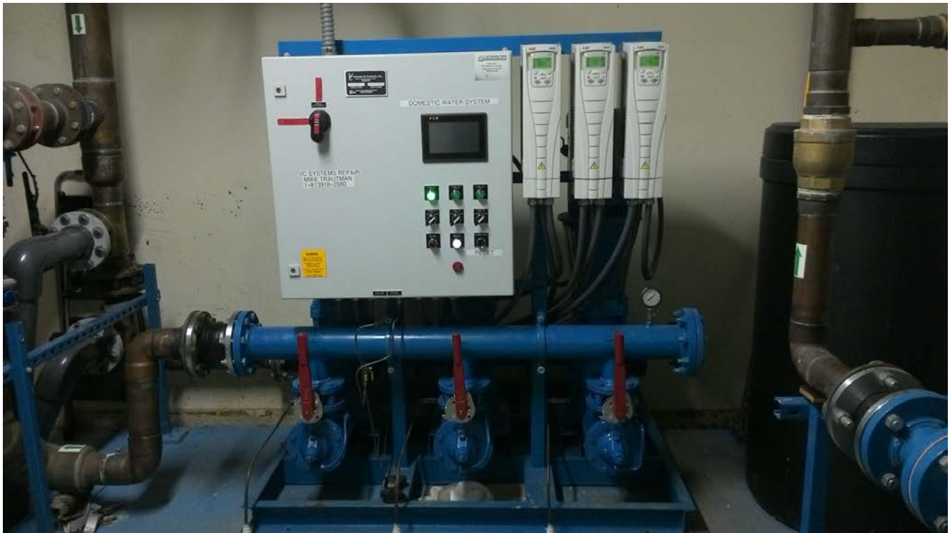
Domestic Water Pumps
