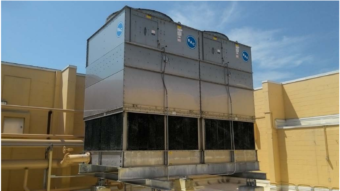
A/C Cooling Tower
