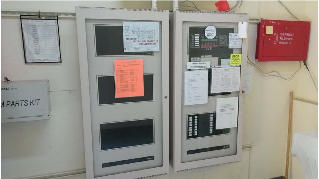
Fire Alarm Control Panel
